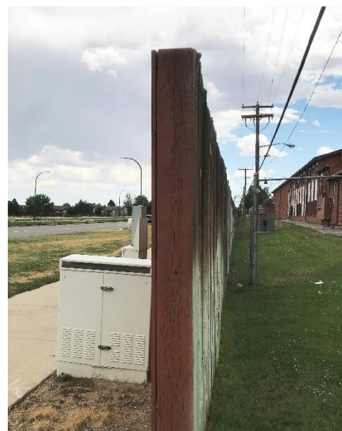
Photo 1: Existing Noise Barrier
